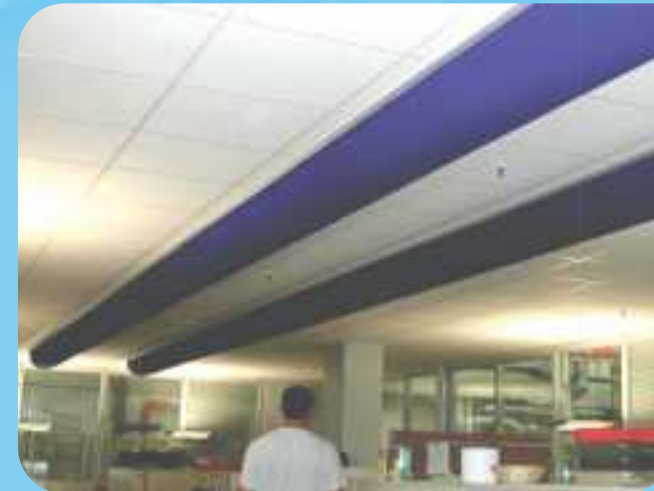
TEXTILE DUCT OFFICE
