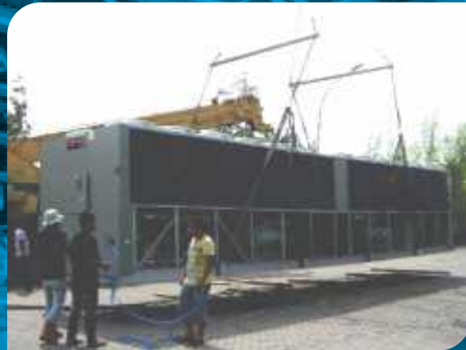
AIR COOLED SCREW CHILLER
