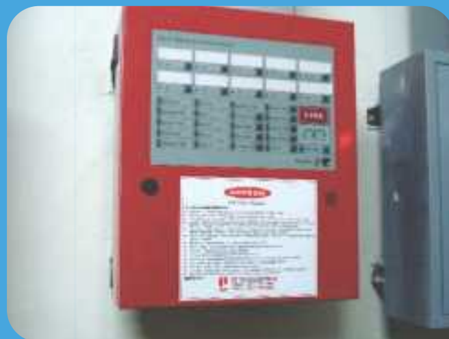
FIRE ALARM SYSTEM
