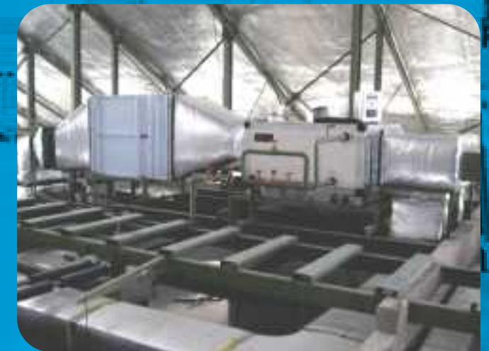
AHU CLEAN ROOM
